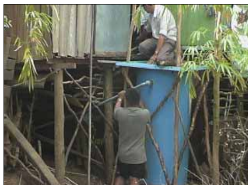
Installation of a piloted Water Flush Floating Latrine in one Flooded Commune of Dong Thap Province
