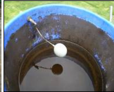
UNICEF Colombia: water storage tank
