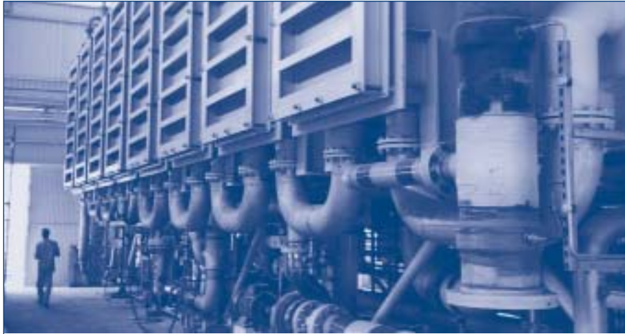
Fig. 18.2. Multi-effect distillation plant with vapour compression (MED +VC) in Mindelo, Cape Verde (capacity: 2400m 3 /day) (photograph by Jan C. Schippers)
