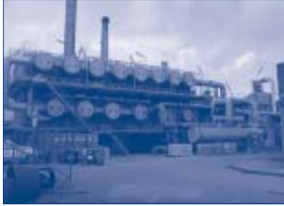
Fig. 18.4. Multi stage flash (MSF) distillation plant, Las Palmas, Gran Canaria (capacity: 2 \times 9,000 \text{ m}^3/\text{day} ; commissioned in 1980) (photograph by Jose M. Veza)
